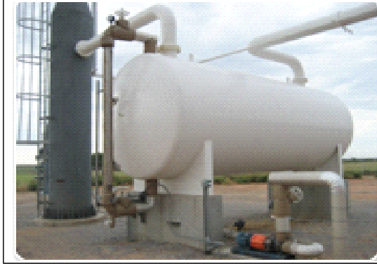
녹아웃드럼 (Knock out drum)
